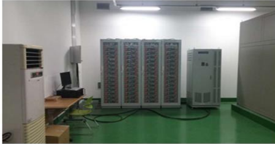
ESS (For KEPCO's 29 branches)
